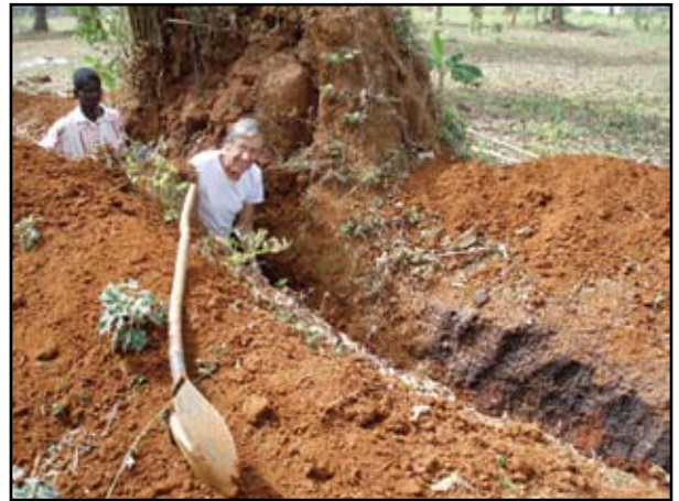
Jack putting in the sewer line...Just call him Art Karney (The Honeymooners)...at least the teams will be able to flush the toilets!
